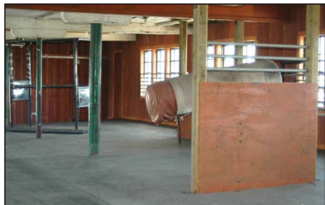
The interior of the horse barn has newly remodeled wood-paneled walls and rubber floors throughout.
